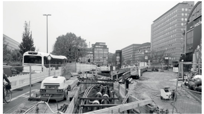
Abb. 2 District Heating pipe trench, Hamburg
