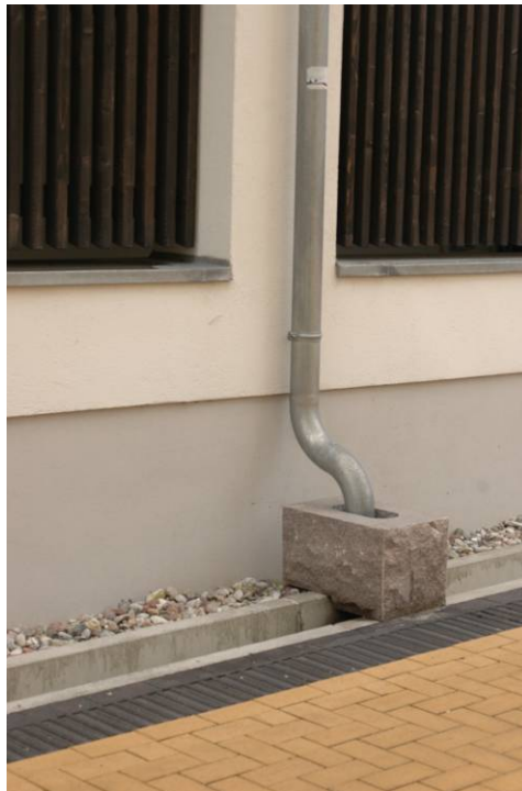
Fig. 9. Debris filter canal in Malmö, Sweden (© L. Kronawitter)
